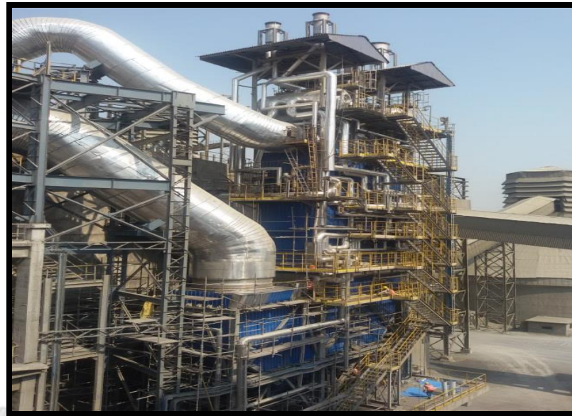
Air-Quenching Boiler (AQC)
