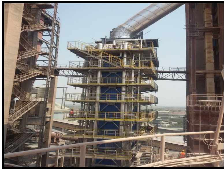
Suspension Preheater Boiler
